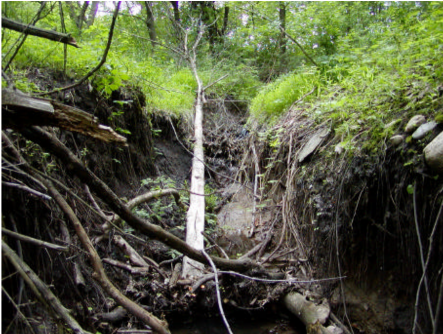
Wetland H channel erosion
