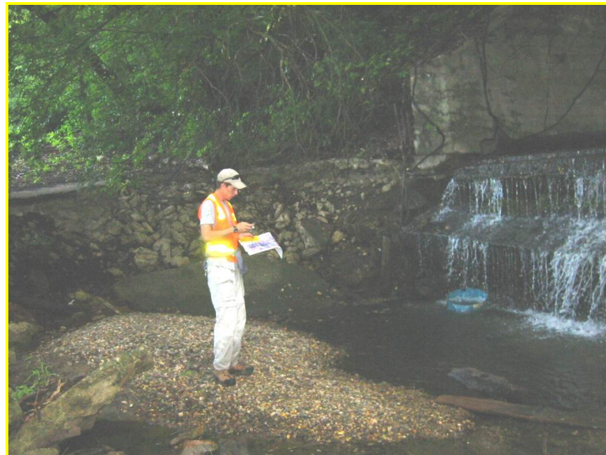
Figure 28 Large drop at downstream end of regional trail culvert
