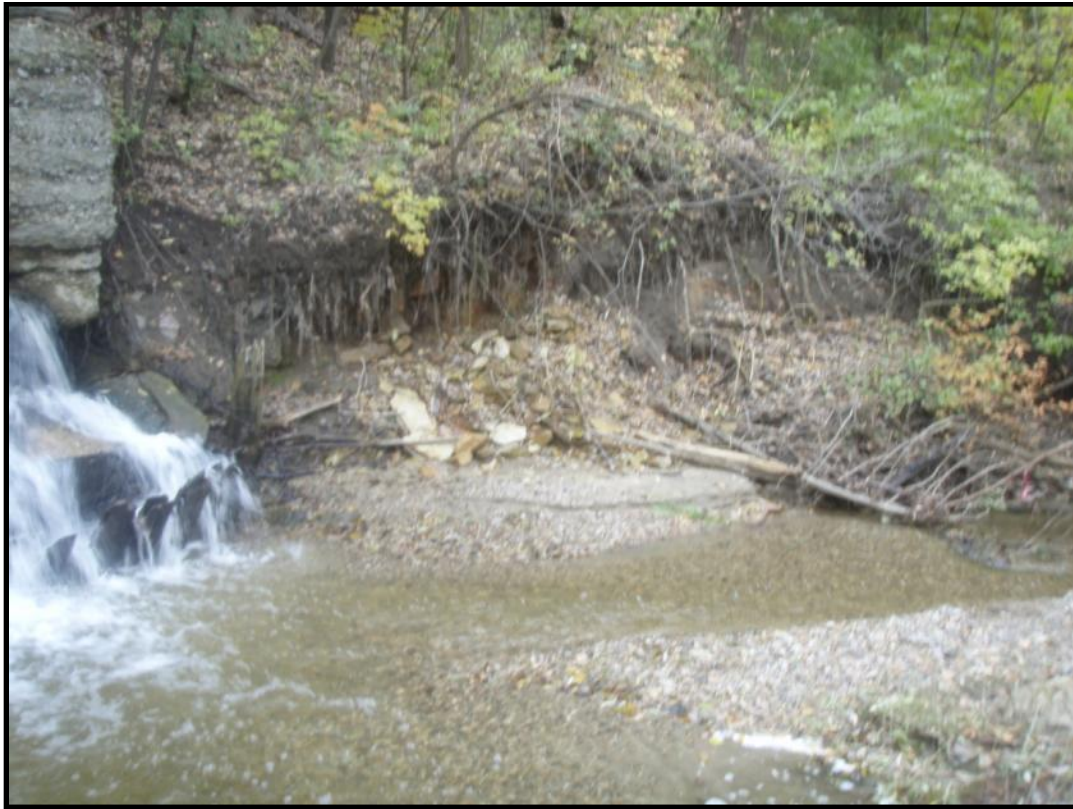
Figure D.8 Eroding left stream bank immediately downstream of culvert outlet
